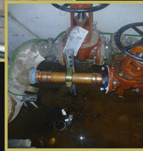
Water Main Break at UHS
